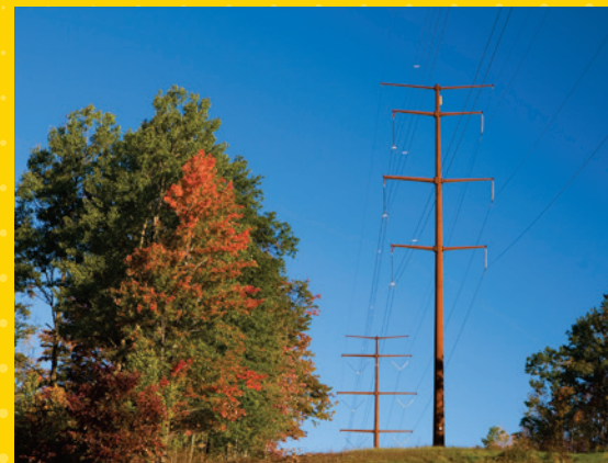
Now: An ATC transmission tower.
