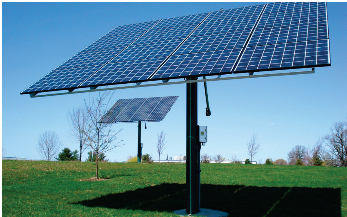
Solar photovoltaic technology installed at WPPI's operations and office facility.
