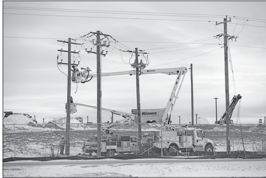
JOE TIMMERMAN/WISCONSIN WATCH Southern Lakes Newspapers Construction unfolds at the 350-plus-acre Beaver Dam Commerce Park, the site of a Meta data center, Jan. 20, 2026, in Beaver Dam. A battle has developed over who will construct the latest in Wisconsin's power grid, needed for the data centers going up.
